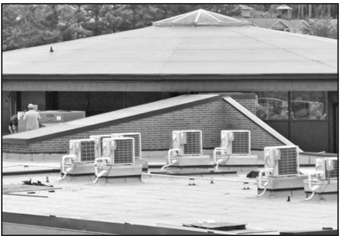
The new roof on the middle/high school building of Towns County Schools has been completed in time for school to start, including all new HVAC units. Photo by Lowell Nicholson
